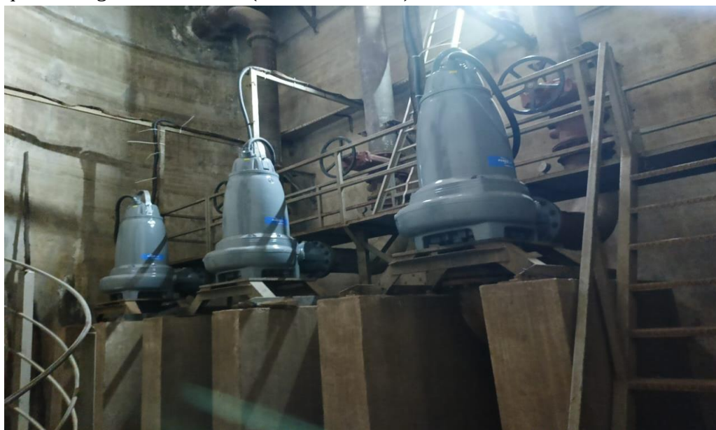
Figure 4: Stations de pompage
